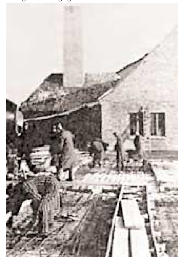
Slave labourers completing the roof of the underground changing room at Crematorium II
